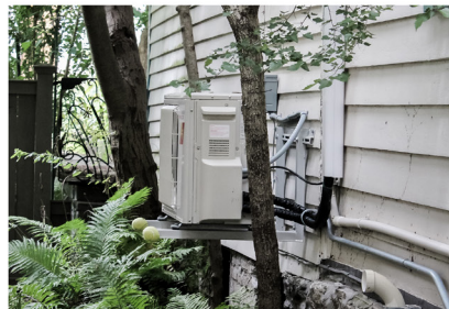
"mounted on the wall" at the side elevation of 420 E Seneca St
