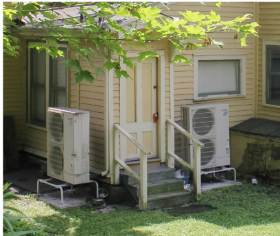
"raised on a platform" at the rear elevation of 522 E State St
