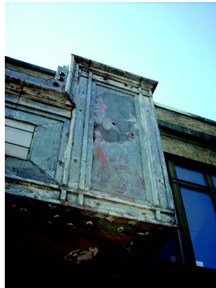
The marquee, seen here scraped down to bare metal, is actually made of Galvaneal, a steel alloy, which is considered by many to be a step up from galvanizing.
